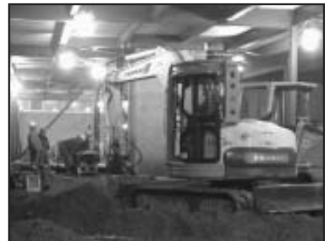
Construction progresses on the first floor of the John Mitchell Center addition.
